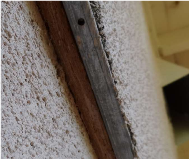
Figure D14: Bark mulch was used in areas at the rear of the home, under one of the decks. Note that the wood-based sheathing product is exposed (lower photograph). Source: IBHS
