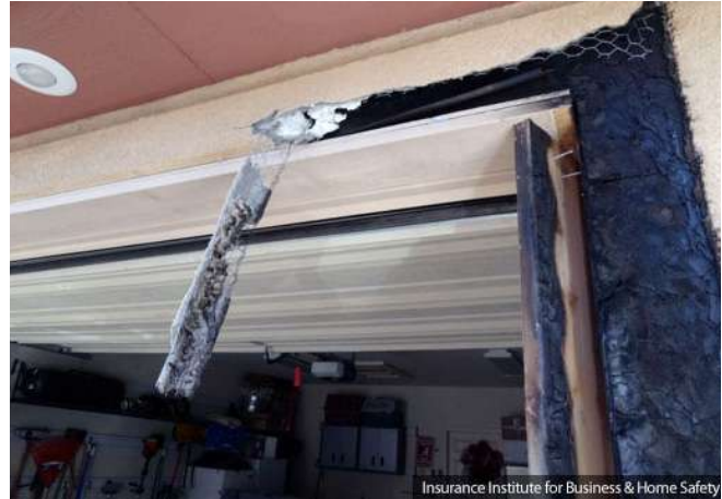
Figure 20: The components of this EIFS system include a noncombustible stucco outer coating, and inner layers of combustible foam insulation, wood-based sheathing, and wood framing. Source: IBHS.
