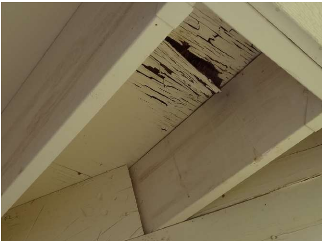
Figure D19: The flagstone covering on this solid surface (noncombustible) deck had failed (upper) allowing water to get below the covering, eventually resulting in fungal decay in the horizontal wood-based sheathing (lower). Source: IBHS.
