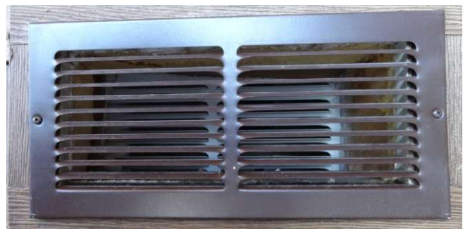
Figure D7: These photographs show venting for the make-up air to a room containing gas appliances. Metal screening was missing from these vents, as seen in the lower photograph. Source: IBHS.
