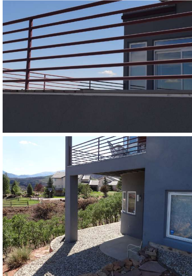
Figure D23: The decks at this home used wood for the structural support system and a combustible wood-plastic composite decking (walking surface) product. Source: IBHS.
