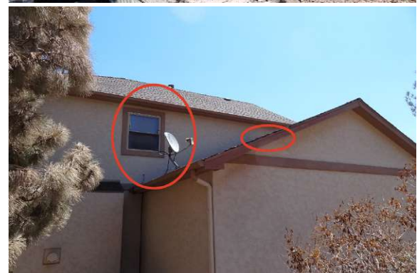
Figure 18: A composite figure of two damaged homes on the west side of Courtney Dr. The up-slope home is above and the down-slope home is below. The charred combustible siding in the up-slope home is not visible in this figure. The damaged components in the down-slope home are circled. Source: IBHS.
