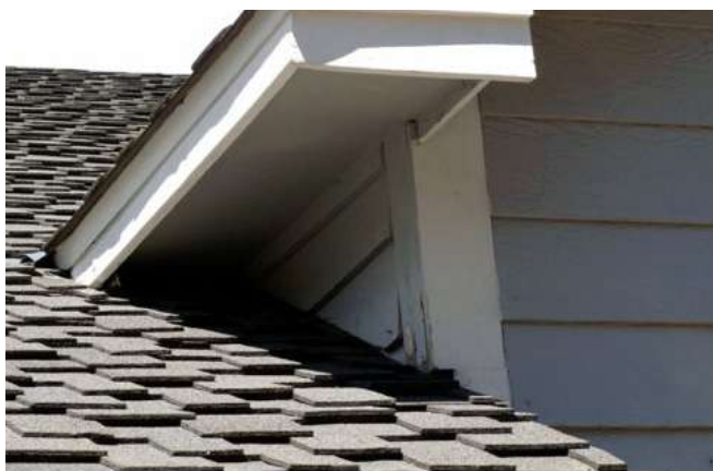
Figure 23: The roof-to-siding return on this complex roof consists of a composite wood (hardboard) siding product and a Class A fire-rated asphalt composition shingle roof covering. Even without vegetative debris at the roof-to-wall intersection, an accumulation of embers could result in ignition of the wood-based siding. Source: IBHS.
