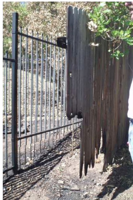
Figure C7: A partially burned cedar privacy fence. Source: NFPA.
