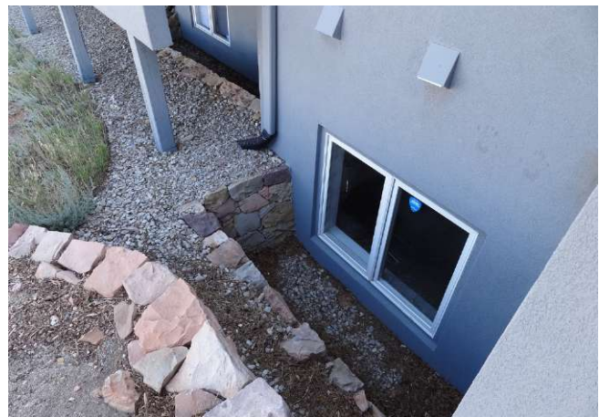
Figure D22: Defensible space in the right side and rear of the home. Source: IBHS.
