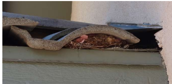
Figure D17: The ends of the barrel-tile roof covering on this home were not “bird-stopped.” Note the debris in the under-roof area at the end of the roof (lower photograph). Source: IBHS.
