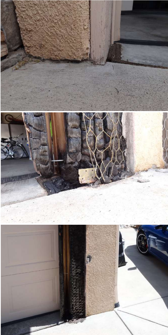
Figure 19: Photographs of the left, middle and right side columns of the two-car garage at a home on Lanagan Street. Note the low clearance between the concrete driveway and the EIFS system, as shown in the left-hand side column. The metal weep screed is visible at the base of the middle column. Source: IBHS.
